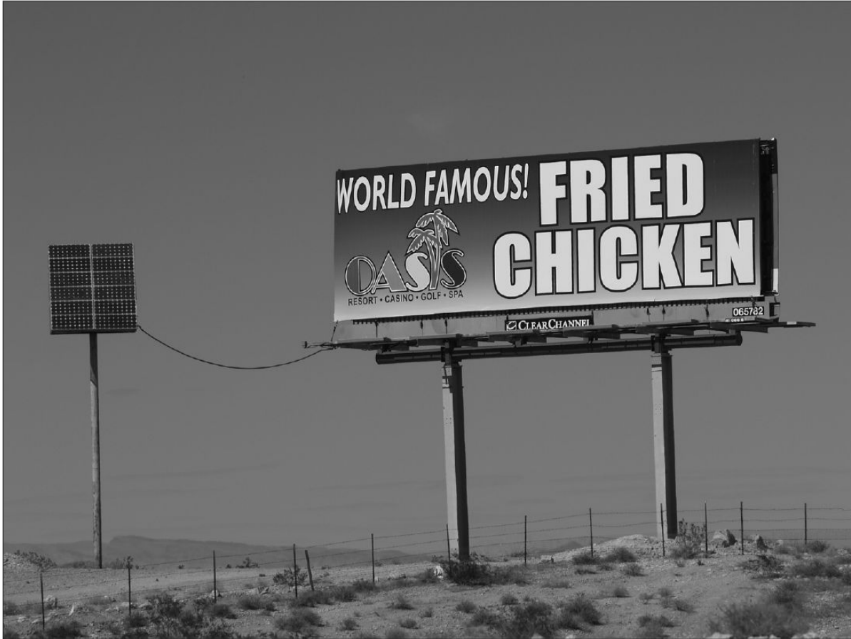
Pole-mounted panels powering billboard lights.
