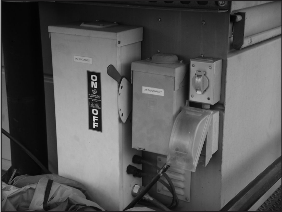
AC and DC disconnects and receptacles, mounted on the rear of the box.
