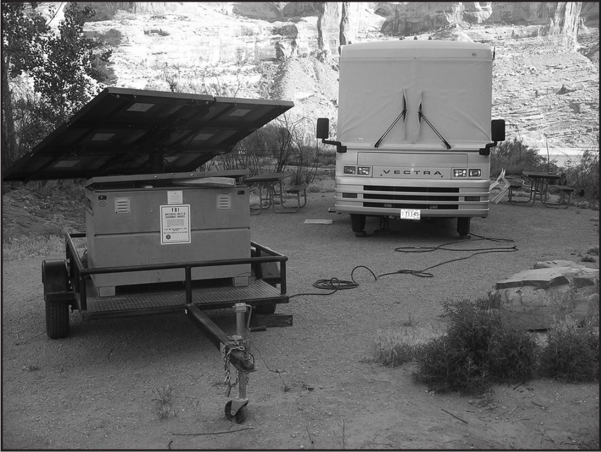
Solar array mounted on a trailer. Note the ground wire leading from the system and spiked into the earth near the trailer hitch.
